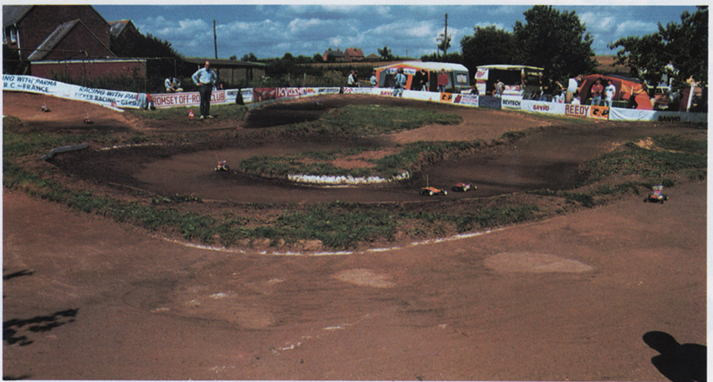
Hard to believe, but true: the light-colored areas in the corner is the result of repairs made with cement! The track surface, as you would imagine, was as hard as cement. Not exactly the proper conditions for a World Class venue.
